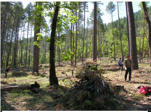
Grayback Forestry personnel completing the 'finish work' in a commercial unit of Pilot Joe
